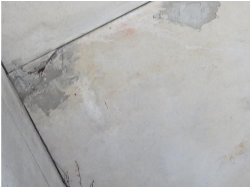
DECK PANEL BAY "A" ABUT. #2 W/ FAILED PATCH
